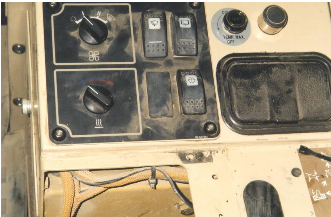
Newer control panel set-up for operator.
