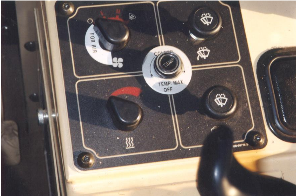
Older style machine thermostat set-up.
