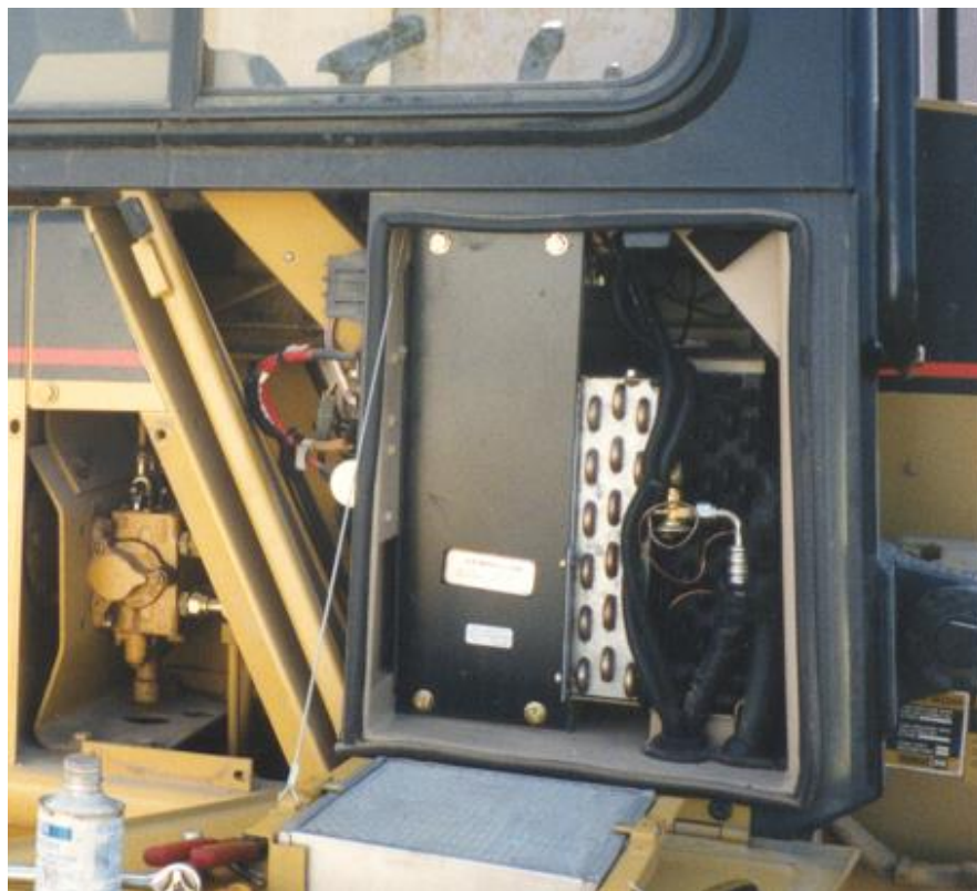
Evaporator assembly in place with lines run.
